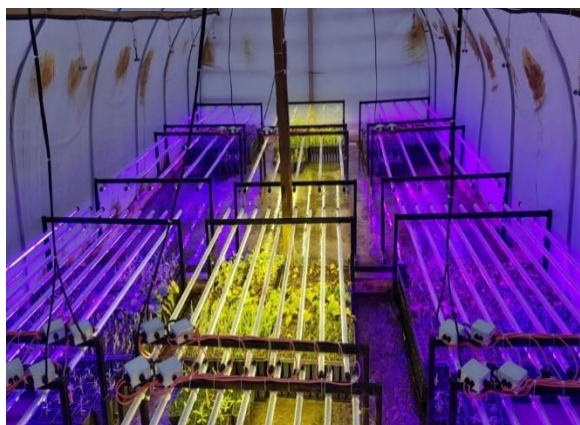
Figure 2. Placement of LED equipment.
